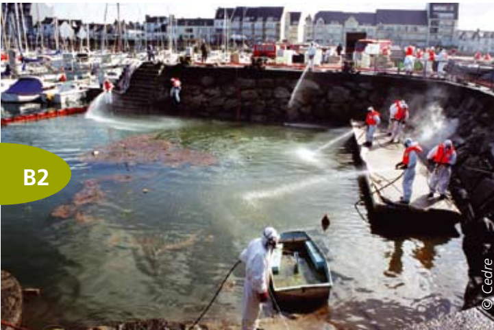
Cleaning riprap and the harbour basin as a result of pollution by heavy fuel oil. Port de la Turballe, France.
